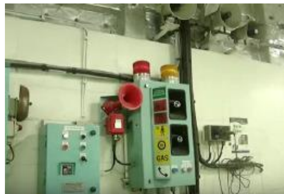
CO 2 discharge alarm in Engine Room
